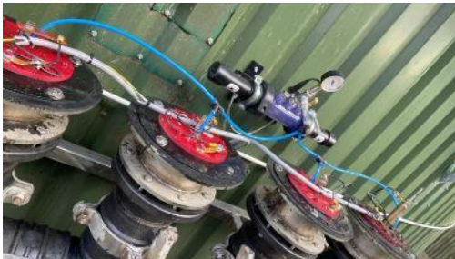
Pictures: Electrolysis electrodes in the feed pipe of the post-digester at partner B.E.S.
